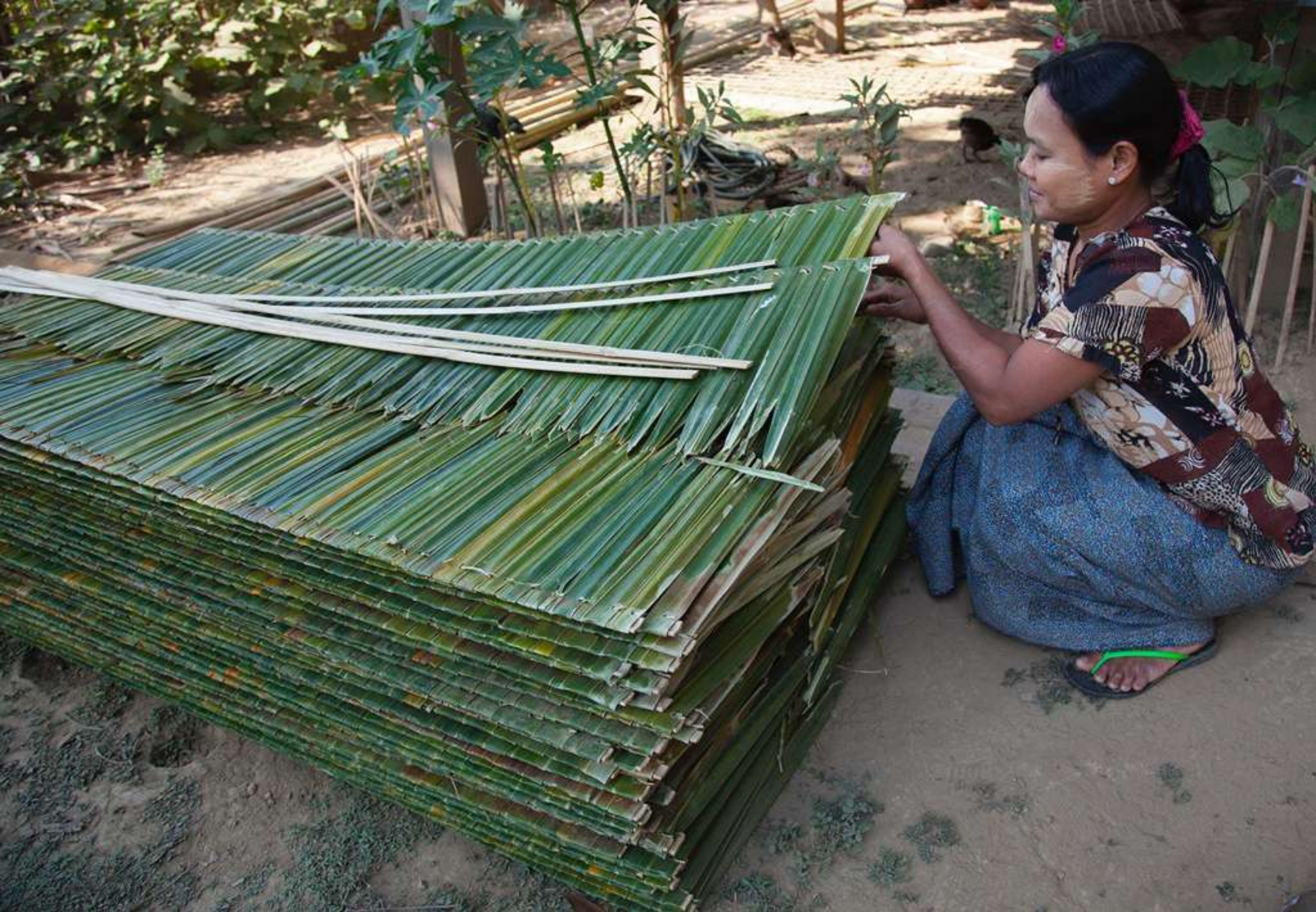
This woman is rebuilding her roof which was burnt by the mob. She is building the new one from palm leaves since she can't afford a metal roof.
